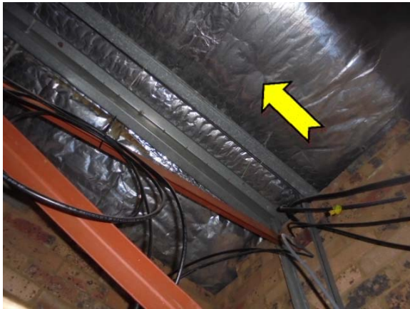
Photo 3. Interior, level 1, loft, ceiling – suspected SMF sarking insulation.
