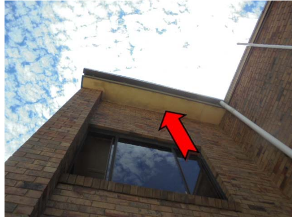
Photo 2. Exterior, north and south elevations, eaves – suspected asbestos-containing fibre cement sheeting.
