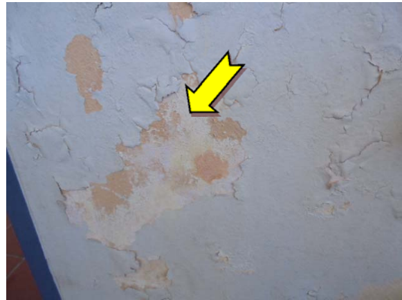
Photo 4. Interior, throughout, walls – suspected lead-containing white lower paint system.
